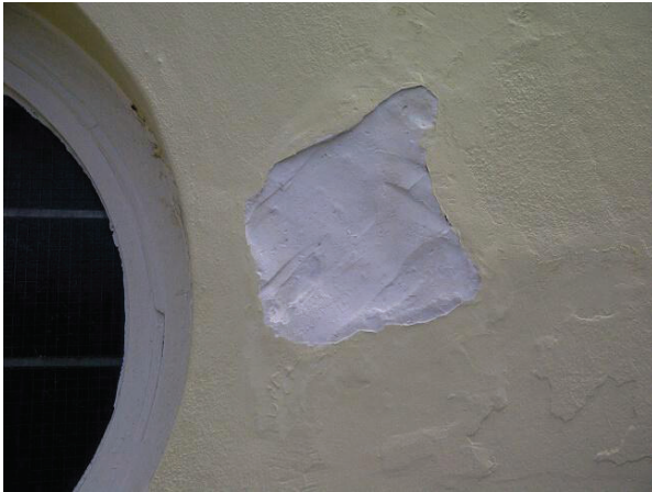
Plaster & paint falling off the building again.
