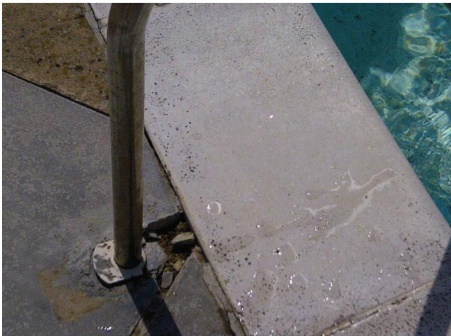
Swimming Pool steps in poor state of disrepair, Crumbling away from the concrete with large holes.
