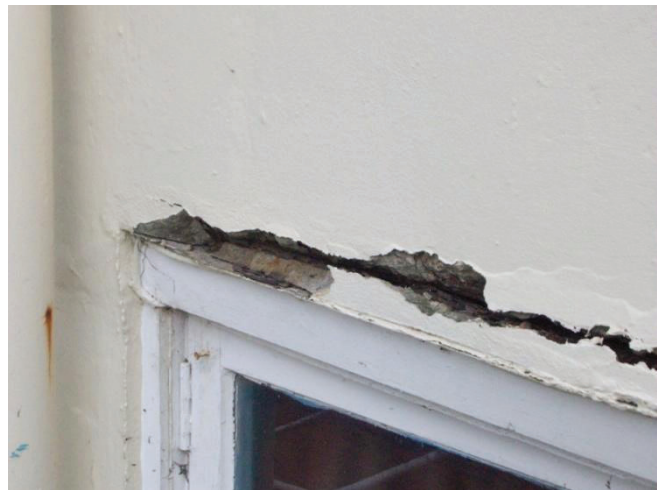
Cracks to exterior of building since disguised with paint.
