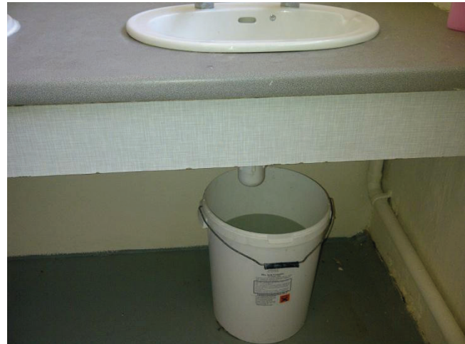
Ladies toilets at the lido. Unclean & with buckets of water to catch leaking drips from unmaintained sinks/toilets.
